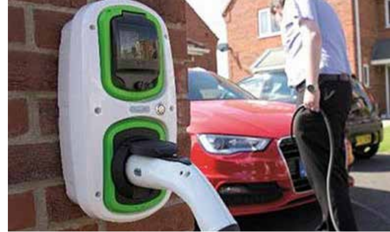
Figure 135: EV charging point (source: Adobe Stock)
