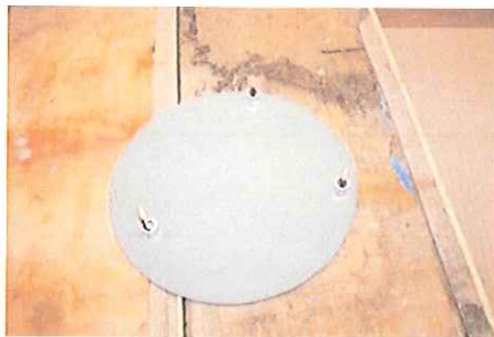
Image showing screws from plaques to building
